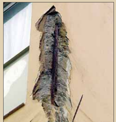
Concrete spalling on the KwaZulu-Natal coast – a legacy of poor planning. Too few designers of concrete structures are ensuring that the current building boom does not lead to history repeating itself, says Contest in Durban
