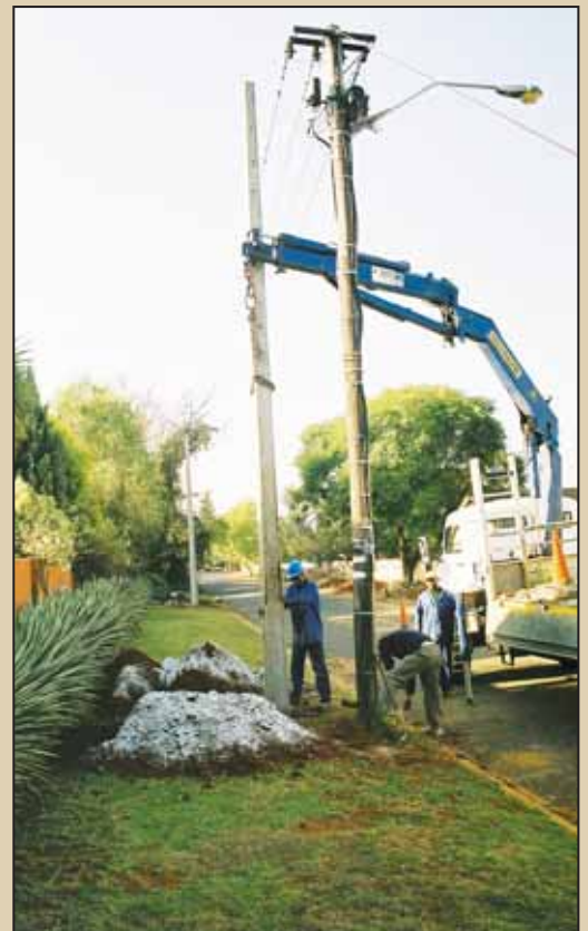
One of 300 prestressed concrete poles supplied by Infraset for a powerline upgrade project in Fairland, north-west Johannesburg, is planted next to the timber pole it is replacing
