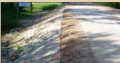
View of the completed road showing the 'concrete block' access, the gravel-filled shoulder, and the SoilSaver-covered side slope section
