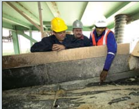
George Hoffmann, Jan Deacon and Mike Mpanza inspecting a polyurethane liner recently installed by Uretech on vibrating feeder VF02 in the secondary crusher screen plant
