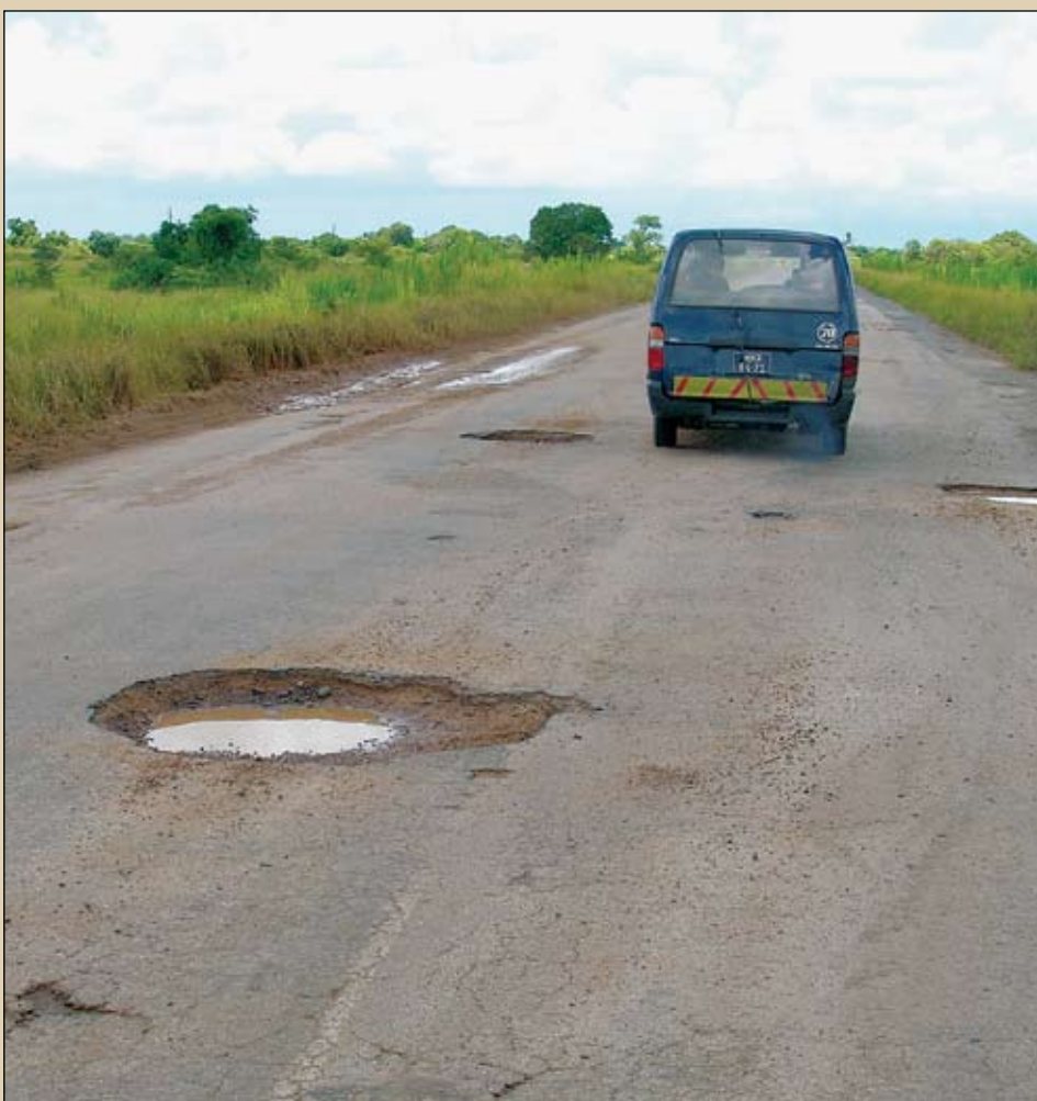
Poor maintenance has led to hazardous travelling conditions on large sections of the EN1. The rehabilitated surface will enhance safety along this section of the route
