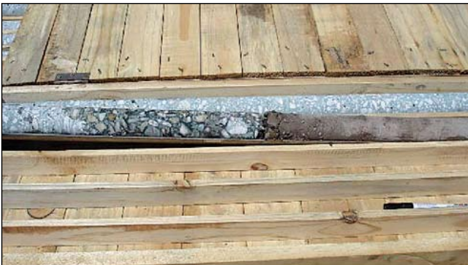
Figure 9 Pile contact on B6/4
