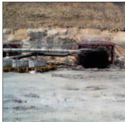
One of the four parallel tunnel entrances at the base of the adit excavation
