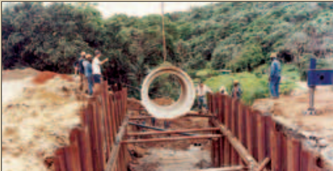
Trench support for 1 800 mm dia stormwater pipe. Depth of excavation 5,5 m (Ballito, KwaZulu-Natal)
