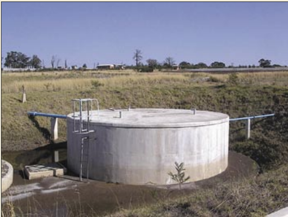
Construction of 100 kℓ leachate tank to collect leachate generated by the waste cell
