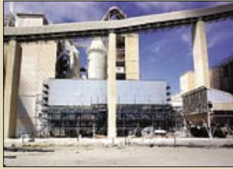
Seen here while under construction by MikroPul is the kiln baghouse of Kiln No 3 at Holcim South Africa's Dudfield plant
