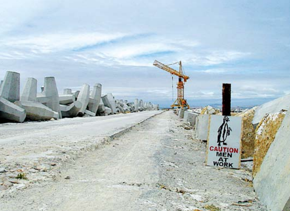
► Left: Construction yard on the island Right: Repairs of the main breakwater are under way Insert below: Construction of the new T-jetty. Extension of the main breakwater in progress in the background
