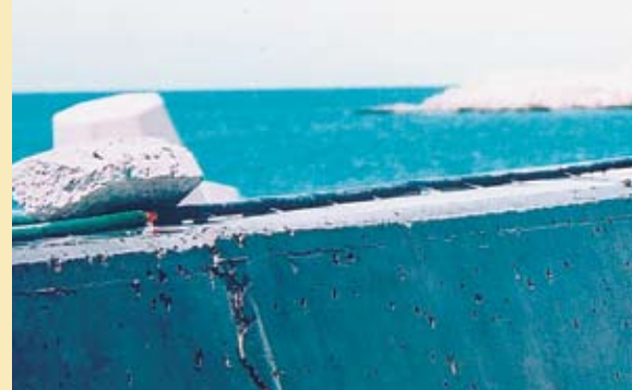
▶ Hosepipe with holes at Coega
