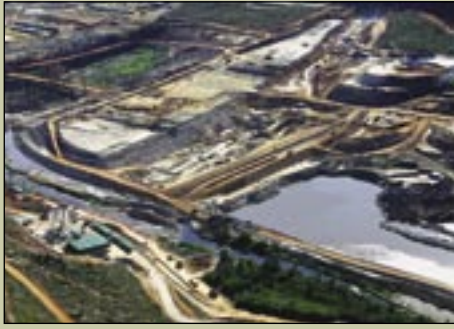
Dam construction on the right bank of the Berg River. The diversion channel is visible below left, behind the crane. The plinth is visible between the cofferdam and the main embankment. The borrow area is filled with water (right)
