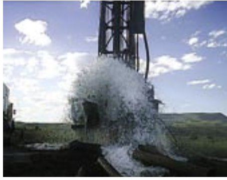
Rotary air percussion drilling in progress at the site where the find was made
