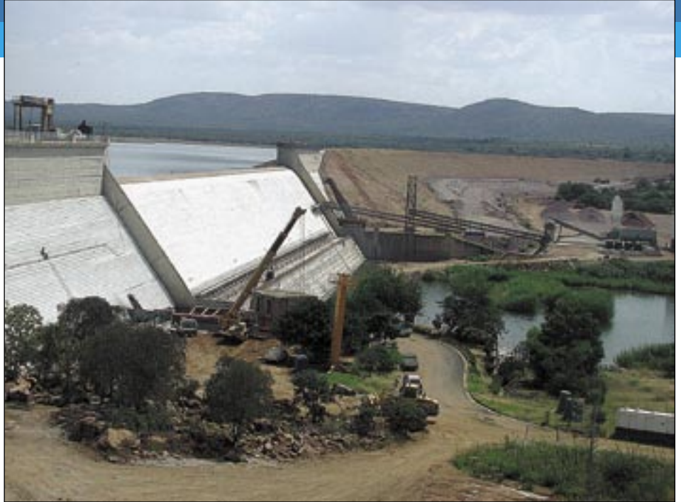
The Flag Boshielo Dam in the Olifants River on the border of the Limpopo and Mpumalanga provinces is being raised to accommodate mining needs in the region
