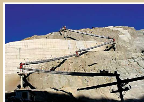
Rotec delivery conveyor system
