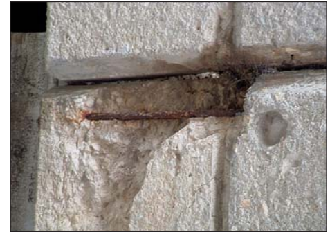
Corroded re-bar resulting in the 'spalling off' of the concrete cover
