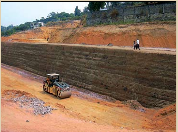
► Top: Filling of gabions at Selembao Bottom: Six metre high Green Terramesh wall
