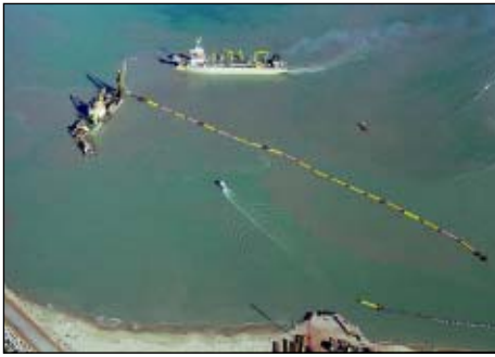
The cutter suction and trailer hopper suction dredgers working in the basin
