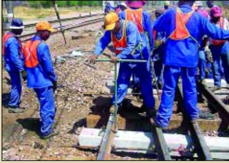
Infrasets Infrabolt steel bolts are torqued to 250 Nm at the Capital Park rail turnout test site in Pretoria. Infrabolt is a patented bolting system specifically developed by Infrasets for the re-engineering of turnouts on timber sleepers with concrete sleepers
