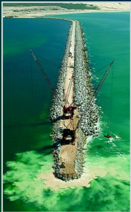
Main: Dolos being stored on the western reclamation prior to placement Insert: The eastern breakwater head under construction
