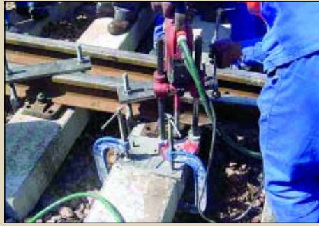
The drilling of bolt holes for Infrasets patented bolting system, Infrabolt, takes place at a rail turnout test site at Capital Park in Pretoria. Clamps keep the rails securely in place while a special Hilti drill is used to drill holes through the reinforced concrete sleeper
