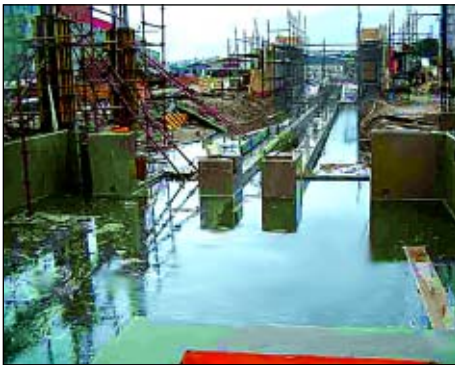
Some problems had to be overcome during the construction of the building ...
