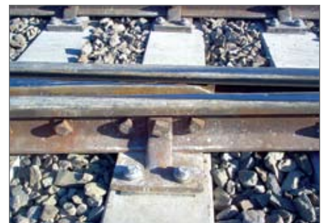
► Above: Timber sleepers which formed part of a turnout prior to being replaced by an Infraset Universal/Infrabolt sleeper turnout set Right: A close-up view of a Universal/Infrabolt concrete sleeper system which replaced a timber sleeper system on this turnout
