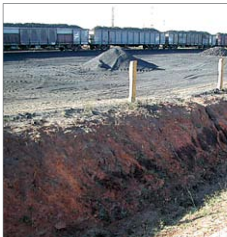
▶ Left: Rietkuil siding prior to siding and loading construction Right: Bulk earthworks for new siding at Rietkuil station
