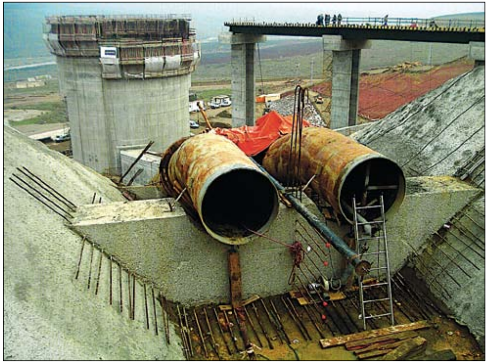
The Athmania system will form part of the Beni Haroun water transfer scheme in Algeria
