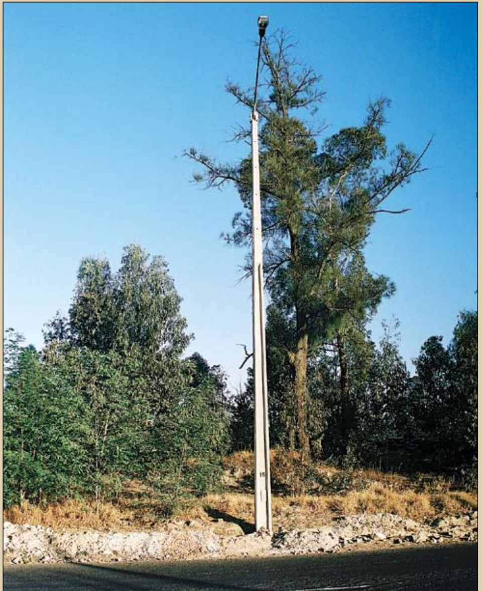
One of the new Infraset concrete poles at Knights in Germiston. The poles were installed as a countermeasure to the cable theft which had been prevalent in the area
