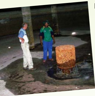
▲ Reservoir Outlet: Due to leaking outlet valve, water drains back from other reservoir.
